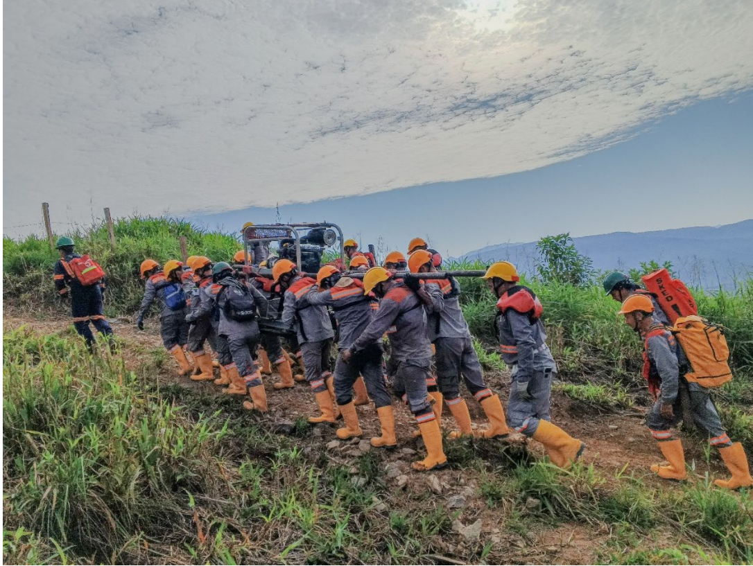
Figure 2 - Man-portable drill rig motor taken up the hill at the Mocoa project
